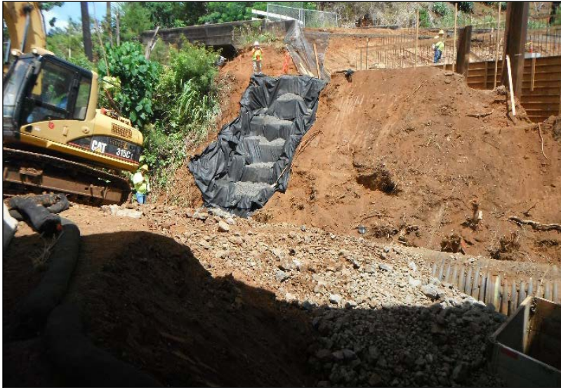
Image Source: State of Hawaii Department of Transportation, Highways Division, Construction Best Management Practices Field Manual , 2021.
