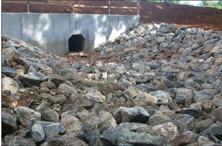
Image Source: State of Hawaii Department of Transportation, Highways Division, Construction Best Management Practices Field Manual , 2021.
